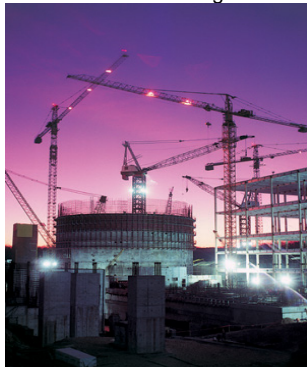
Fig. 3 – A construction site is hazardous
