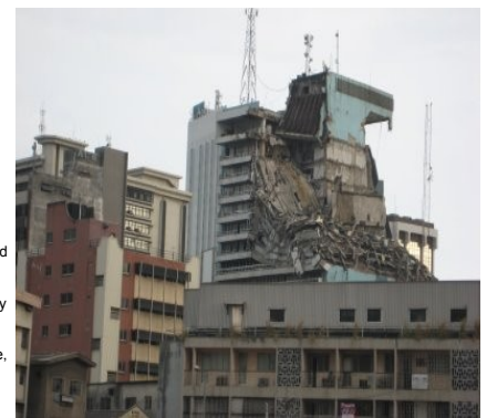
Figure 6: Collapsed Building in the Central Business District in Lagos Source: TJS Blog—Morocco, West Africa, Mozambique
